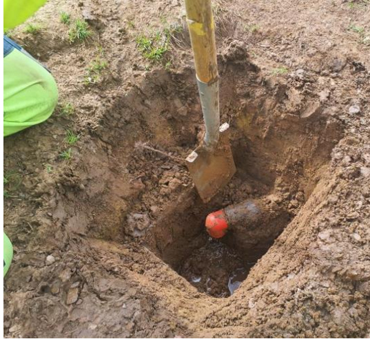
Figure 3 – Buried air valve
