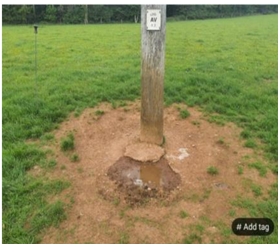
Figure 1 – Air valve chamber as found
